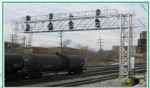
New Signal Bridge
